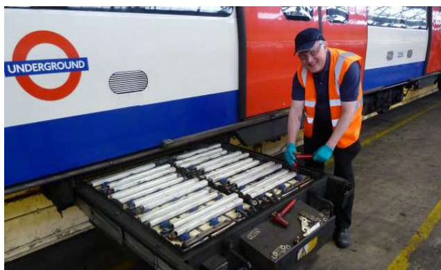
Saft onboard batteries on Alstom’s London Underground Northern Line metro trains
