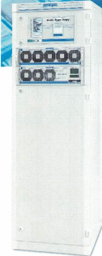
Fig. 8: Inverter- rectifier cabinet with: 3 inverter modules, static and manual bypass Total AC output power 4.5kVA 5 rectifier modules output voltage 220V DC, output current 50A DC
